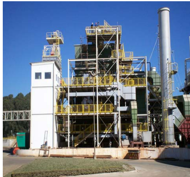
Fig. 4—Picture of the case study boiler at Araucaria.
