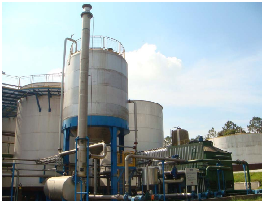
Fig. 3—Dedini's demonstration plant.
