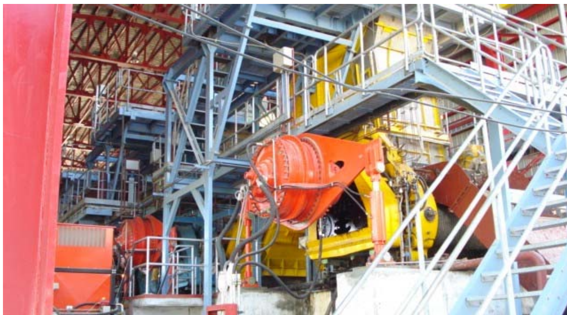
Fig. 2—Juice extraction milling plant with shaft mounted hydraulic drive.
