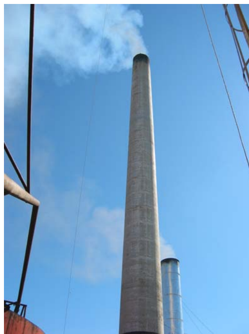
Fig. 5—Santa Clara boiler stacks after post combustion implementation.
